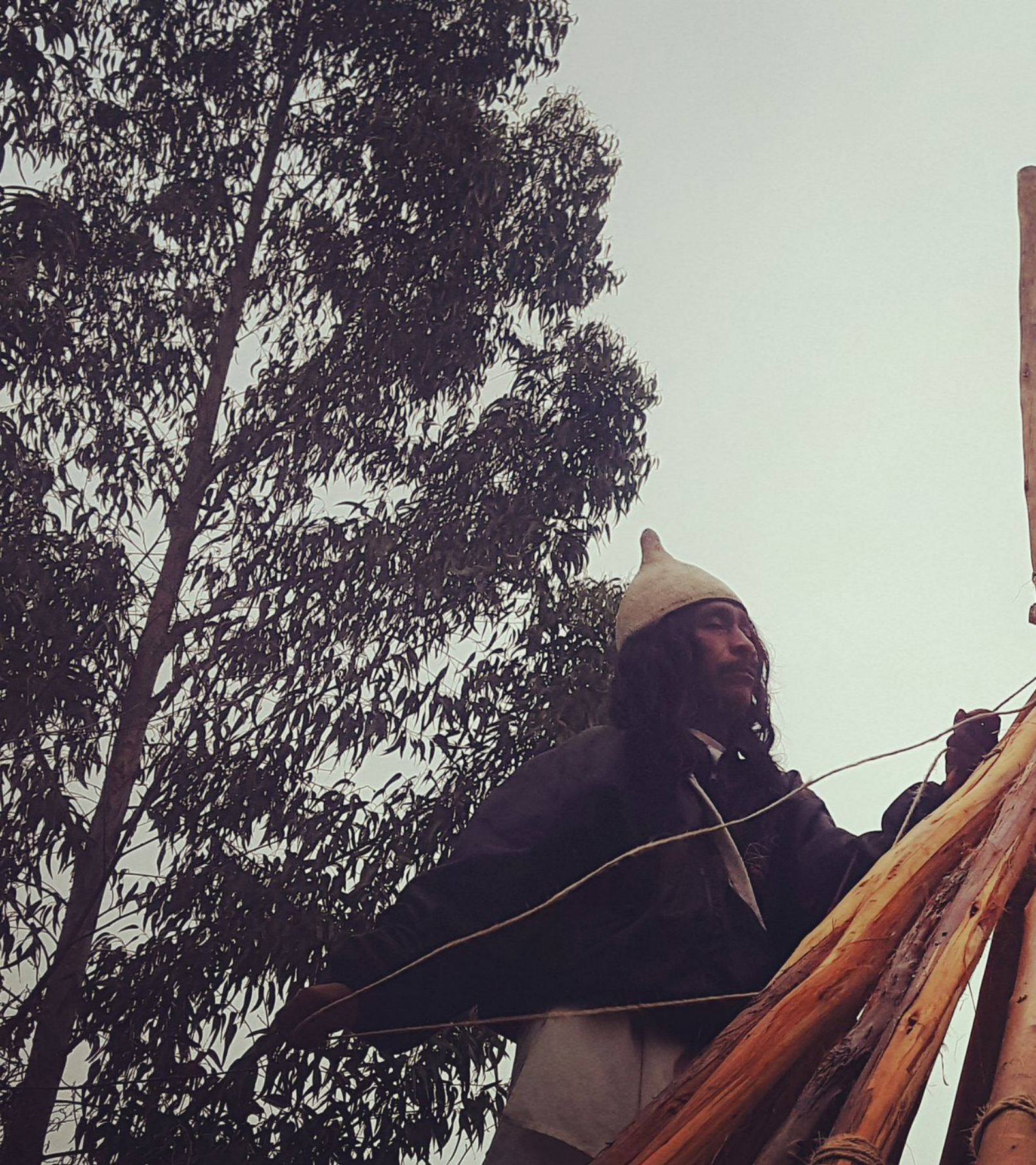
..... Above: Constructing the maloca at Organizmo, Colombia. The process of construction is as important as the structure itself. (Image: Organizmo)
