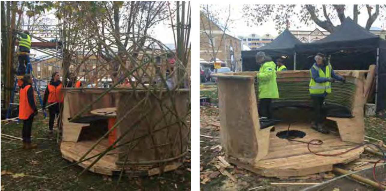
Figure 4: Construction of the pods - dome (left) and interior cladding (right). Images: Helen Norrie.
