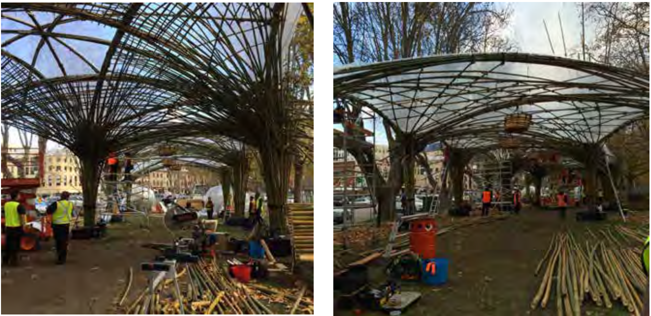
Figure 5: Roofing complete on central bay (left) and end bay (right). Images: Helen Norrie.
