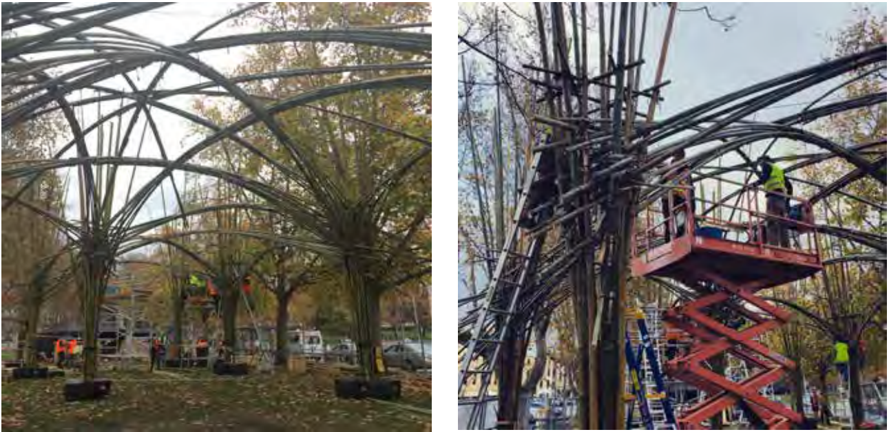
Figure 3: Central bay of canopy (left) and column and beam junction. Images: Helen Norrie.
