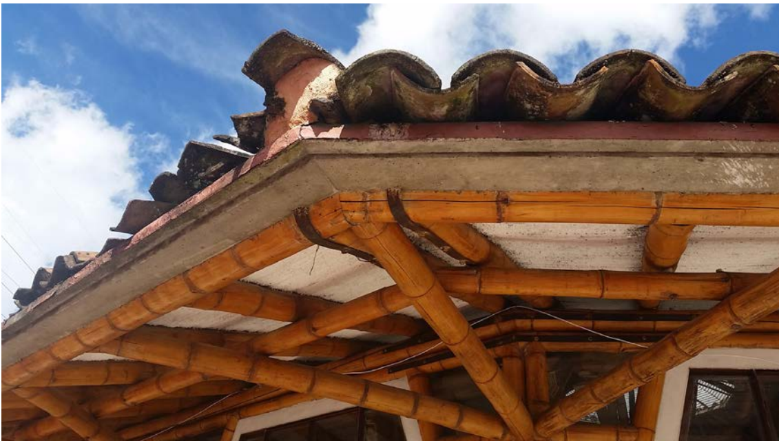
Simon Velez pour's a thin concrete layer atop his bamboo roofs to combat uplift from wind loads Manizales, Colombia Image: Jed Long ▼
